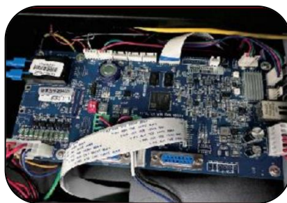
Hoson Control System
